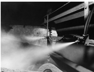
Fig. 5 Two-media nozzles, being a part of spraying installations, reduce dust concentration are installed and directed to the source of dust generation
