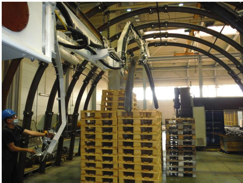
Fig. 7 Ride of the manipulator loaded with the support arch over the roadheader and the operator's cabin (pallet) with the stabilizing foot folded
