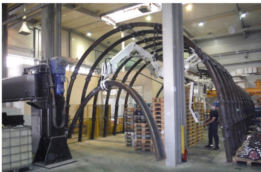
Fig. 8 Manoeuvring the support arch at the support frame installation site, with the use of (unfolded) stabilizing foot
