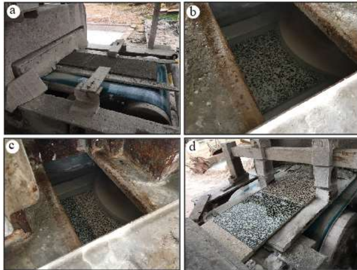
Fig. 4 Production of tile samples a) Removal of sub-base roughness, b) Surface Thinning, c) Surface polishing, d) Final products
