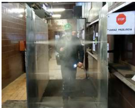
Fig. 12 UMID disinfecting installation
