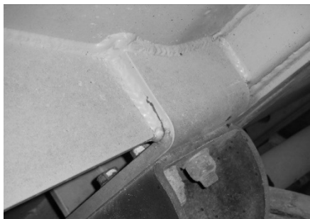
Fig. 1. Crack in the weld
