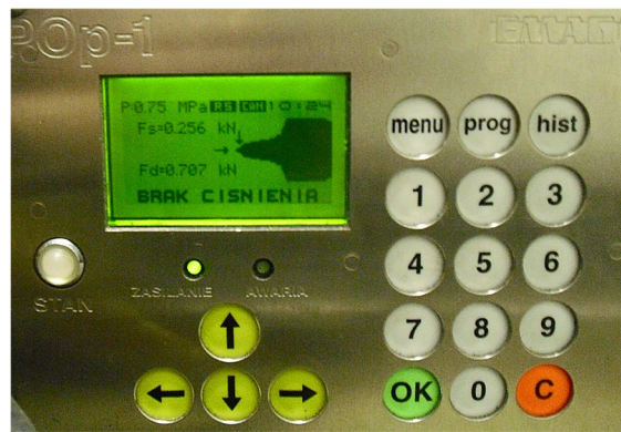
Fig. 15. Operator panel with screen
