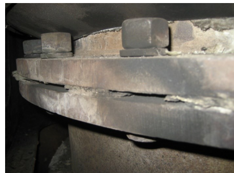
Fig. 2 View of a blown out seal in the connection of the boiler with the exhaust collector of a utilization thermal-oil boiler
